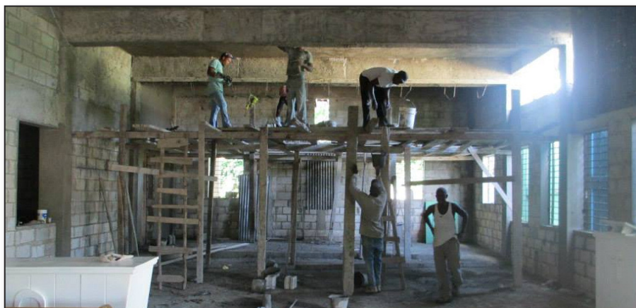
May 2014: Preparing to plaster the walls and ceiling of the first floor.
