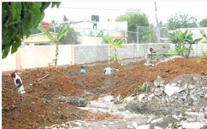
April 2012: The former building has been demolished, and work has begun on the foundation for the new building.
